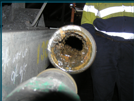
Examples of pipe obstructions causing low pressure within PWCS's process water system
