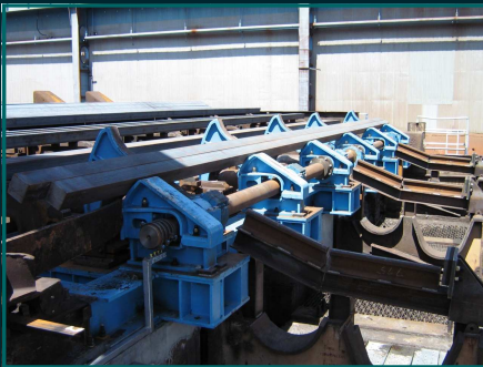
Photo of the final system in operation
